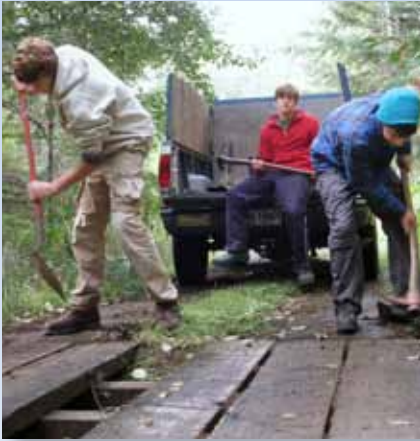
Tenth graders repair the Lousignont Creek bridge at Hyla Woods, during the forestry management block.
